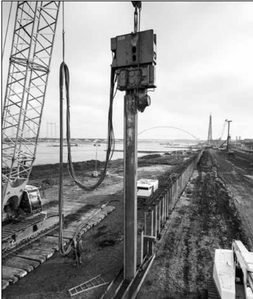
Fig. 11.2. Pitch and drive operation using guide walings at ground level to prevent excessive rotation of piles.
